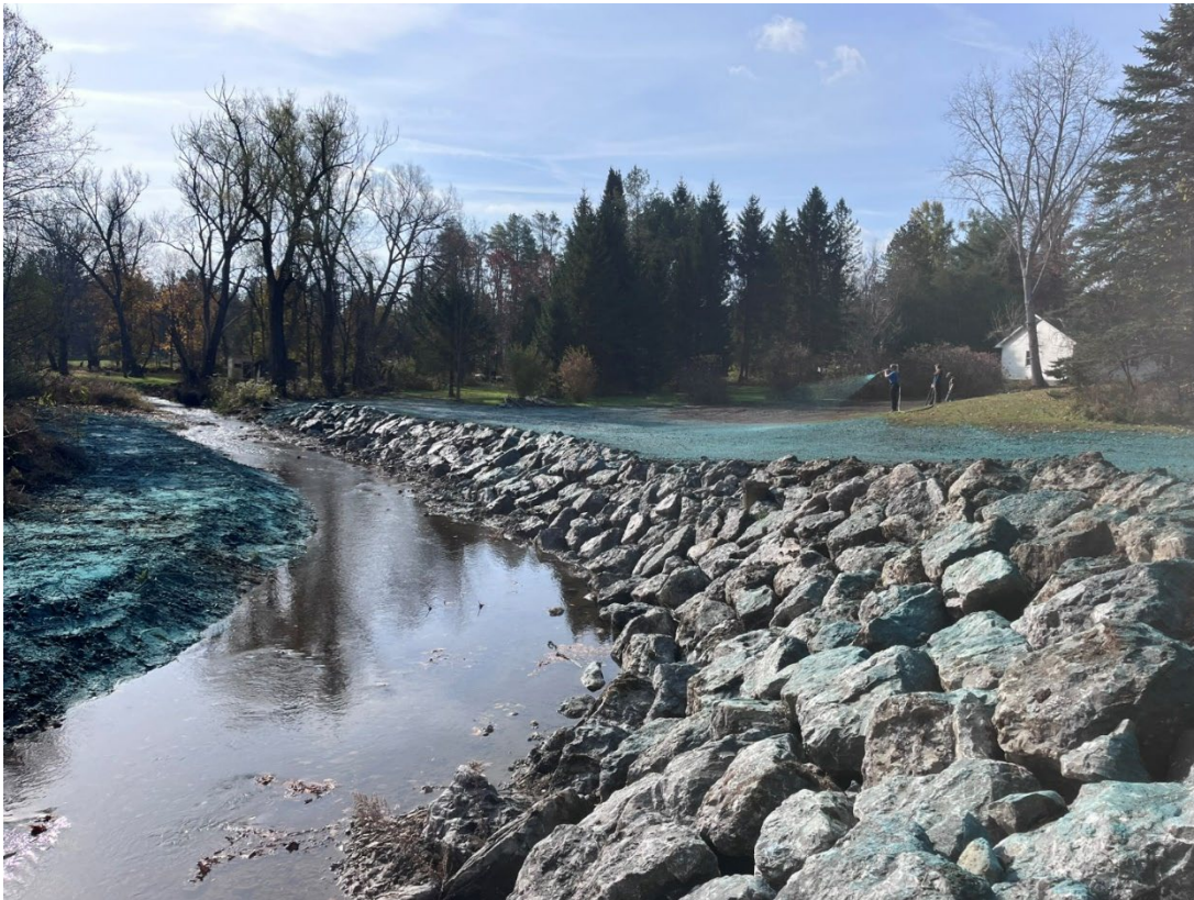
Figure 1. Wyoming County SWCD implemented 350' of streambank stabilization on the Oatka Creek in the Town of Warsaw. November 2024
