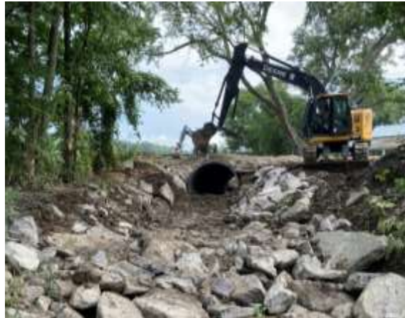
After—Pipe size was increased to improve storm passage. Pipe elevation was lowered to minimize plunge pool at outlet and rock riprap installed to stabilize streambanks and minimize erosion.
