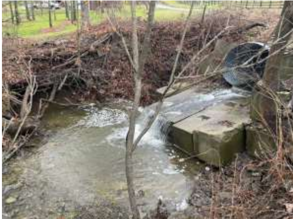
Before—Outlet had 3' plunge pool and severe bank scour.
