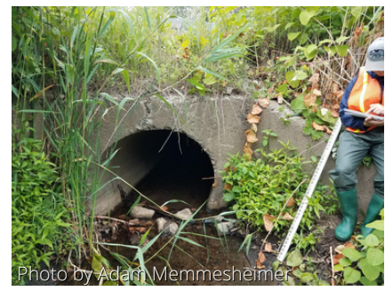
Photo by Adam Memmesheimer (Above) Outlet photo of a round culvert as Gabby logs crossing data
